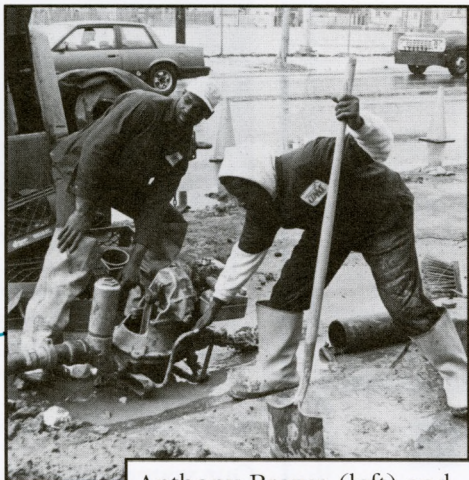
Anthony Brown (left) and Greg Pace (right) of Distribution gather up their equipment after completing an emergency repair to a hydrant line.
