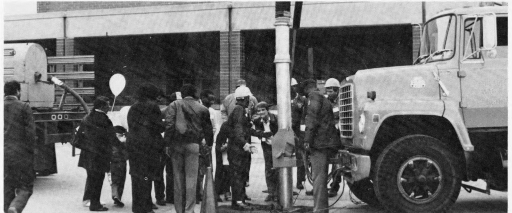
Sewer Maintenance Crew cleaning a sewer at the Southwest Water Pollution Control Plant.
