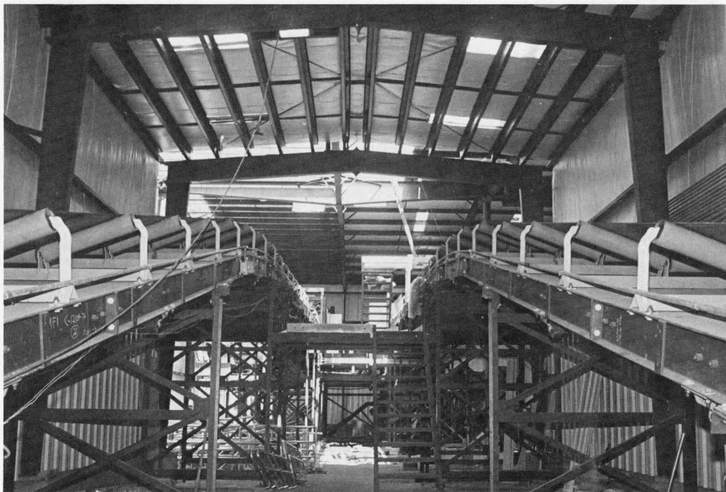
Inside of Receiving/Mixing building showing conveyor belts leading to mixing end of building
