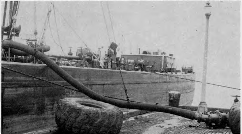
DIGESTED SEWAGE SLUDGE IS PUMPED ABOARD a barge at the Northeast Treatment Works in preparation for hauling of sludge to the Atlantic Ocean.
