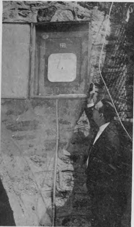
DEPTH OF FLOW GAUGE at sewer outfall in Northeast is inspected by Joseph V. Radziul. The gauge is synchronized with rain gauges in same area, making possible storm flow studies.
