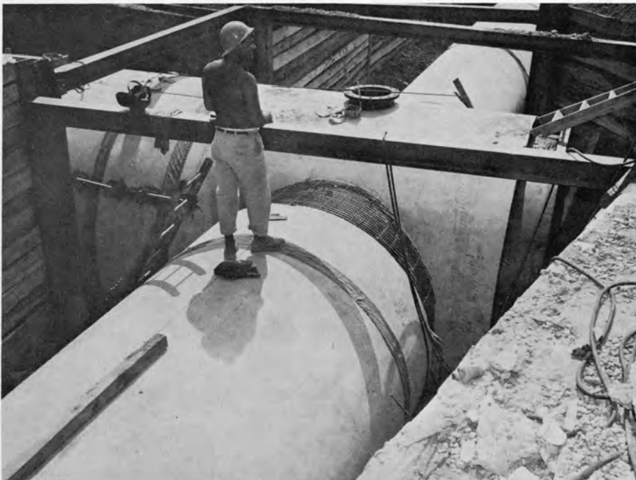
ADEQUATE WATER FLOW to the new basins will be assured by this 11-ft. diameter conduit (center), with first of several planned 7-ft. lines branching from it.
