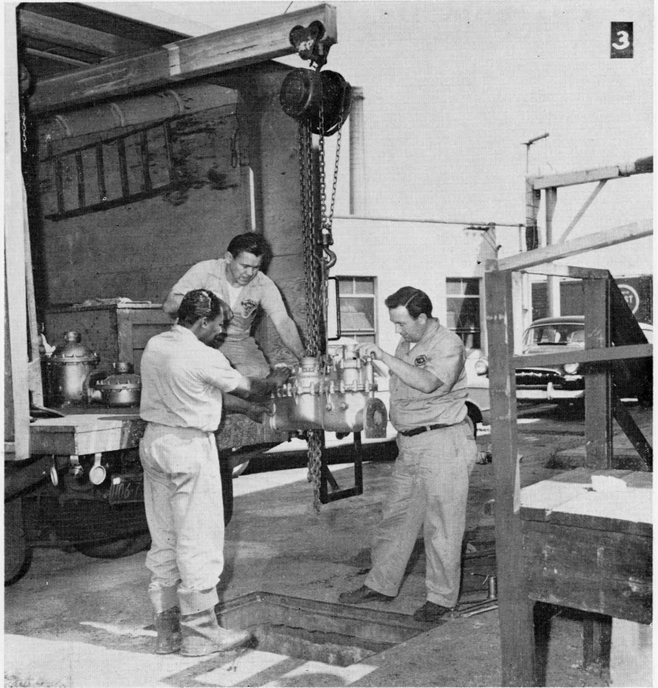
IT'S A NORMAL DAY for Meter Shop crew as a three-inch water meter is replaced at an industrial plant. Photos: (1) Crew consisting of (l. to r.) James Holmes, Lewis Kuriger, and Joseph Kowalski uses large key to shut off water, (2) Holmes removes old meter in pit, (3) new meter is lowered into pit. Crews keep big meters operating, for the big ones produce more than half of all revenue from meters.
