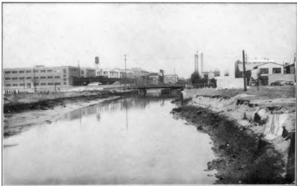
A—LOOKING DOWNSTREAM AT BRIDGE STREET SHOWING SMALL WATERWAY OPENING.
