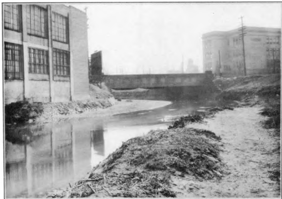
B- LOOKING DOWNSTREAM AT TORRESDALE AVENUE BRIDGE. LOWER SECTION OF WIN- DOWS AT LEFT FILLED IN TO PREVENT FLOOD DAMAGE.
