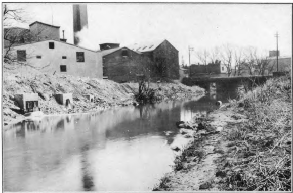
B —LOOKING DOWNSTREAM AT WINGHOCKING STREET BRIDGE. POOR ALIGNMENT AND INADEQUATE WATERWAY REQUIRE RECONSTRUCTION OF THIS BRIDGE.
