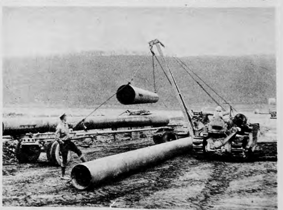
Oil will soon flow through these sections of the "Big Inch" pipeline, shown ready to be put into the trench blasted out of the river bed. Immediately after the blast drilling was resumed for additional explosions.
