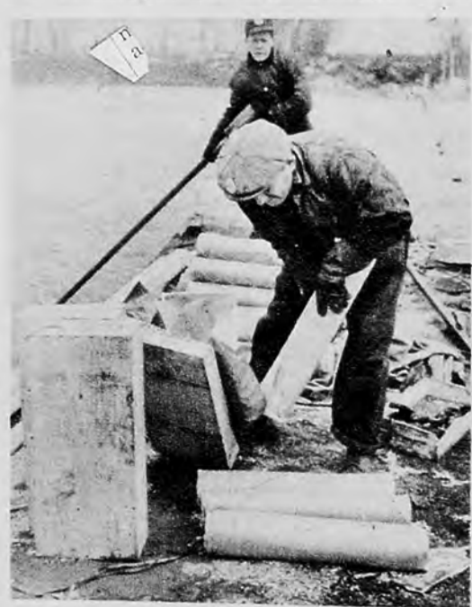
Workmen carefully unpack dynamite cartridges. For the blast, 600 25-pounders were placed in 413 holes in the river bottom.
