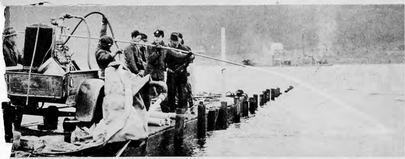
Three weeks were required to prepare for the blast. Here, explosive experts lower dynamite into steel containers which have been drilled into the river bed. In the background is the proposed path of the pipeline across the river.
