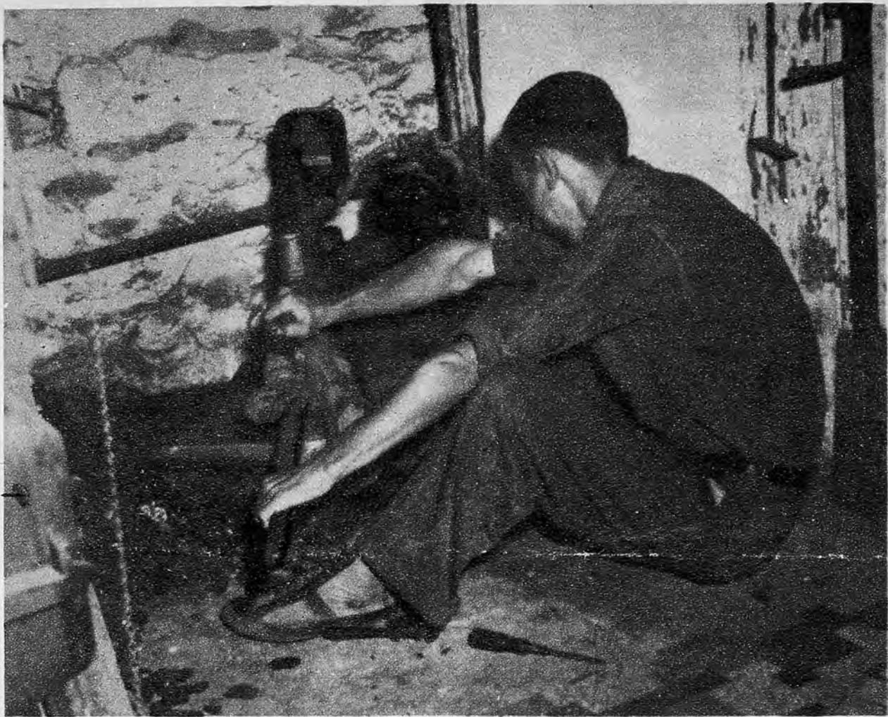
Depressions don't bother Point Pleasant workmen. They shift from one trade to another with alacrity. G. Walton Howarth, town electrician, takes on a plumbing job. He also is a carpenter.
