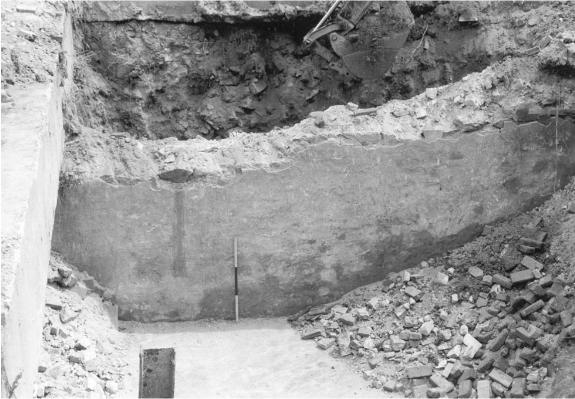
A-17. Interior east wall (plastered) of 529 Market Street basement, showing exposed concrete floor; demolition rubble within 527 Market Street in background, view east-southeast.
