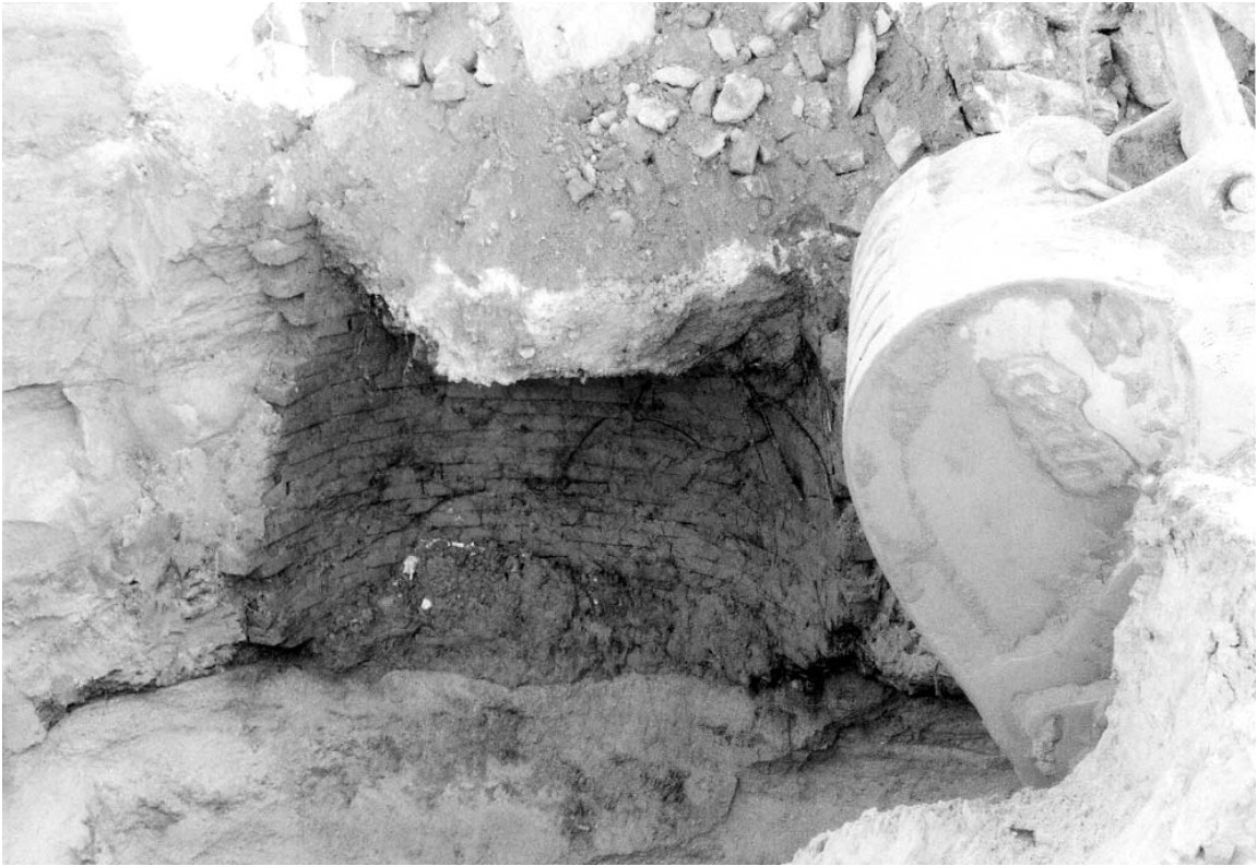
A-9. Feature G (exposed during Phase III shoring excavation) after collapse of its interior fill, view northeast.
