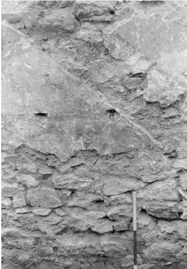
A-21. Stairway scar on interior west wall of 527 Market Street basement, view west-northwest.
