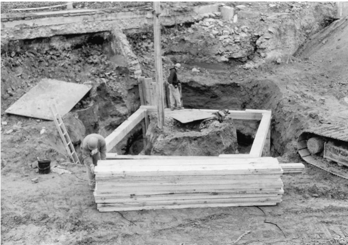
A-12. Construction of wooden shoring box around Feature B during Phase III.
