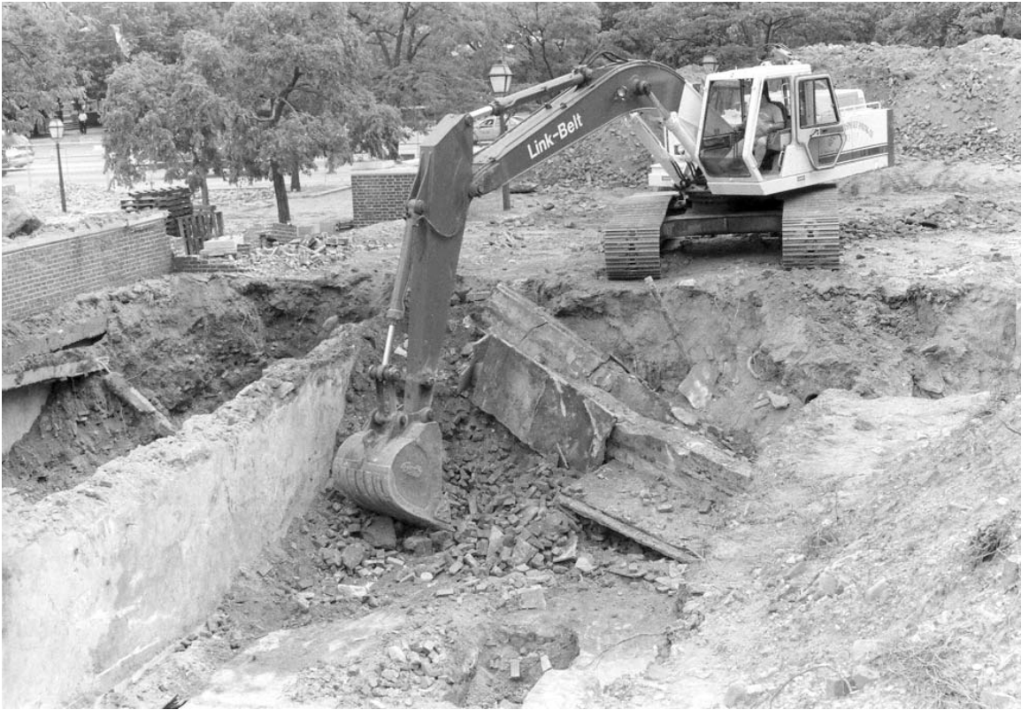
A-3. Link-Belt LS-3400 trackhoe removing rubble from basement of 529 Market Street, view south.
