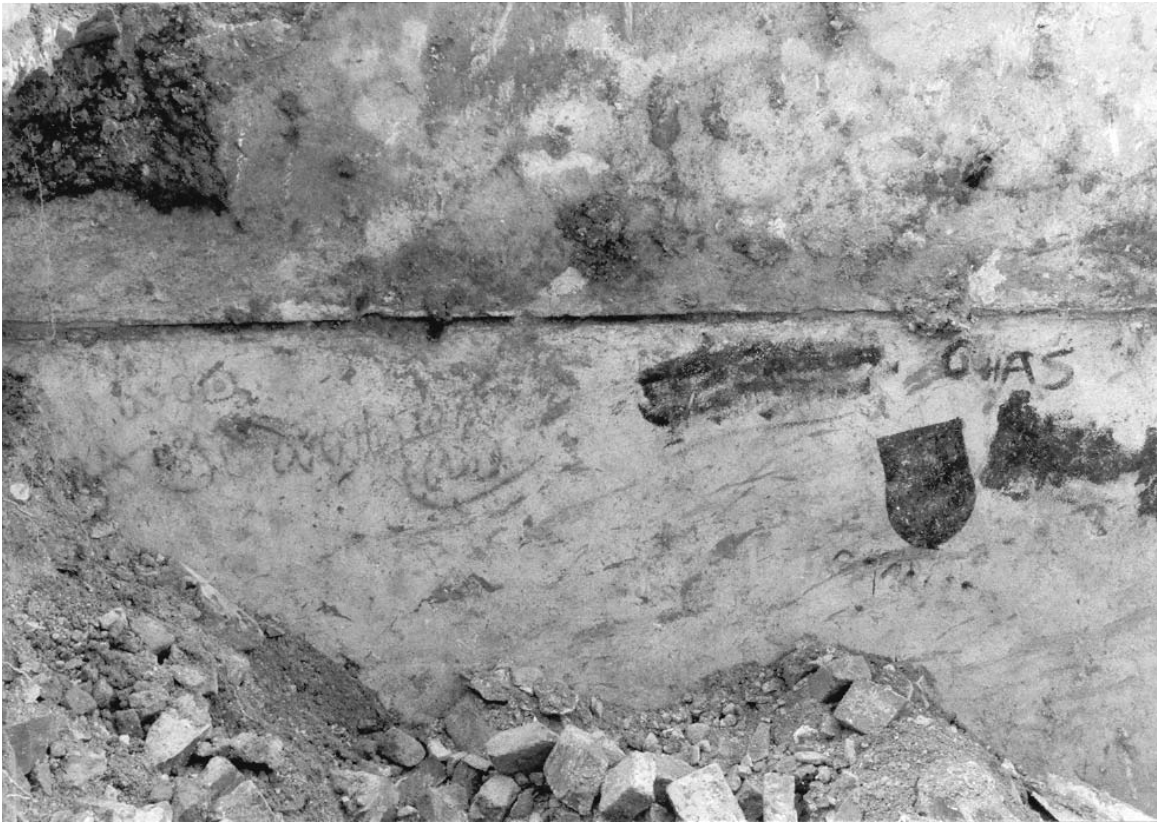
A-22. Graffiti on west interior wall of 529 Market Street basement, view west-northwest.
