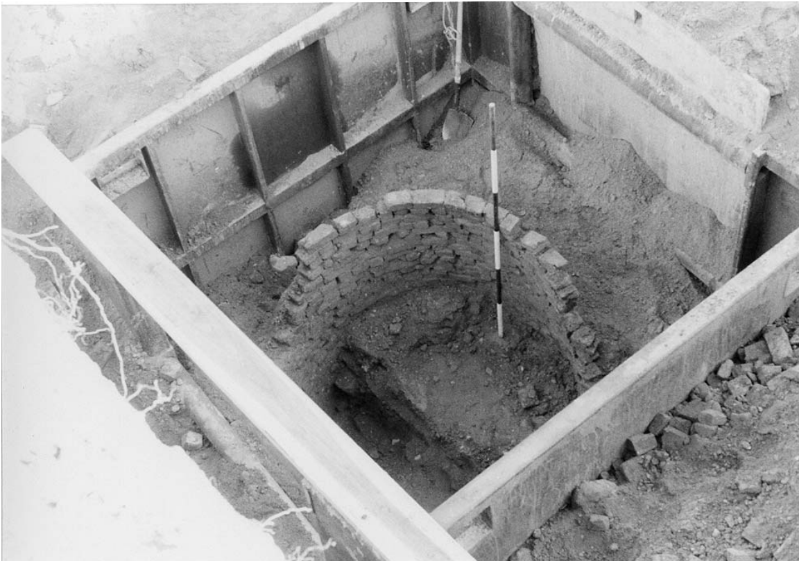
A-6. Steel shoring box placed around Feature A during Phase III, view northeast.
