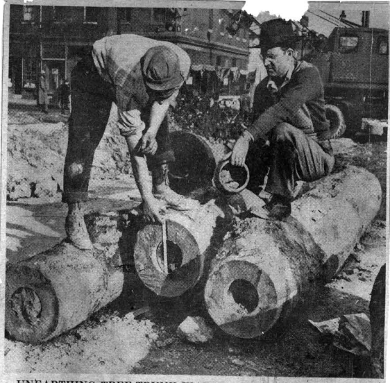
UNEARTHING TREE-TRUNK WATER MAINS ON VINE STREET Frank De Pelipies (left), foreman of a construction crew, and Al Tymna, a city water inspector, looking over the tree trunks which served as water mains under Vine st. for more than 200 years. They were dug up yesterday near 10th st. as work progressed on the Vine st. improvement program. Tymna holds one of cast-iron pipes that served as a connection between the logs. The wood seems unharmed by the long service.
