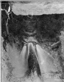
The effect of traffic on a 6" hydrant joint—25,000 g.p.d.
