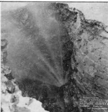
A good trick if it only worked. A sewer manhole found resting on a 6" main cost 100,000 g.p.d.
