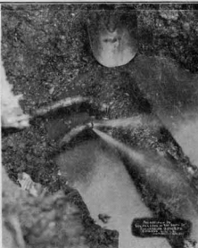
Some of Our "Philadelphia Story" A typical service leak of which there were many—15,000 g.p.d.
