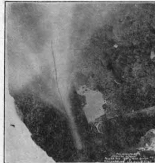
A cracked 12" main shooting away 455,000 g.p.d.
