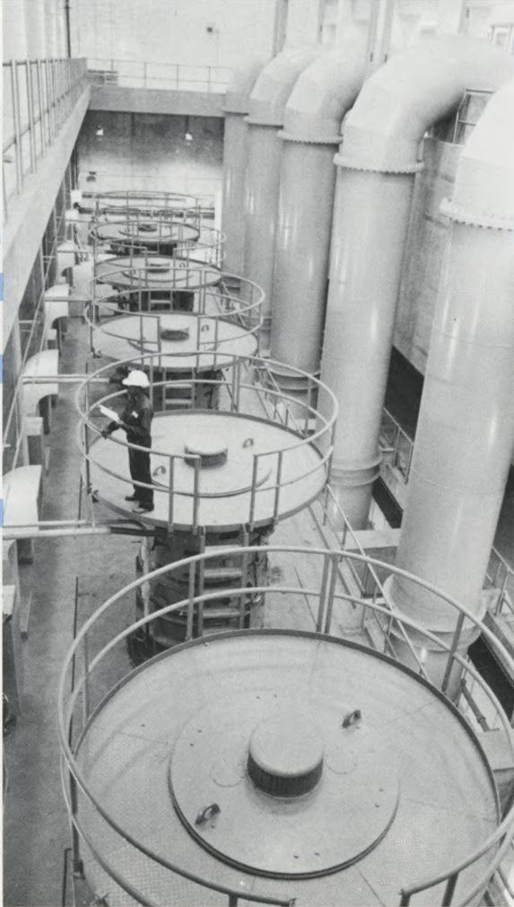
Incoming wastewater from sewage lines in the Northeast are raised by five 85 mgd influent pumps located in the Preliminary Treatment Building of the Northeast Water Pollution Control Plant.
