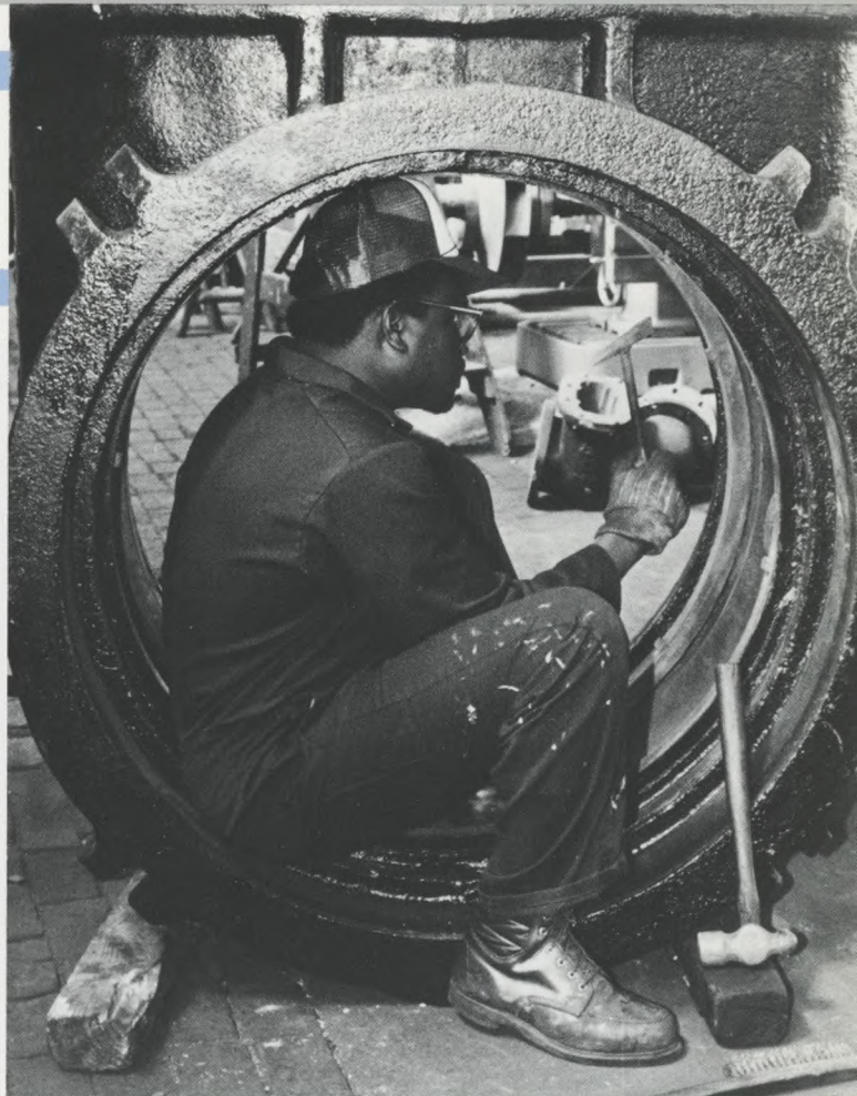
Rebuilding large valves in the Department's Machine Shop yields considerable cost savings.
