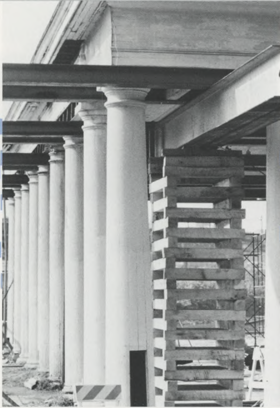
The roof of the Fairmount Water Works Pavilion, which was built in 1871, was raised to facilitate the removal of the huge wooden columns for restoration.
