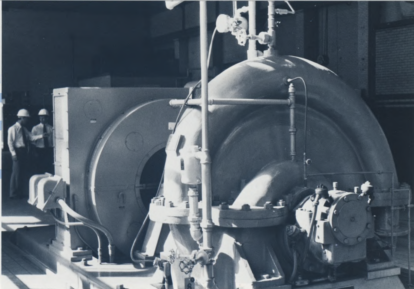
A 2,000 horsepower motor drives this 30 mgd pump at the Belmont Raw Water Pumping Station.
