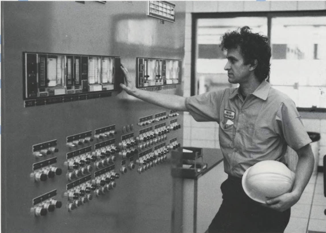
Operator observes Control panel in Compressor Building at the Southeast Water Pollution Control Plant which houses three 9,000 cubic foot per minute air blowers and two 1,000 horsepower multi-stage air compressors.
