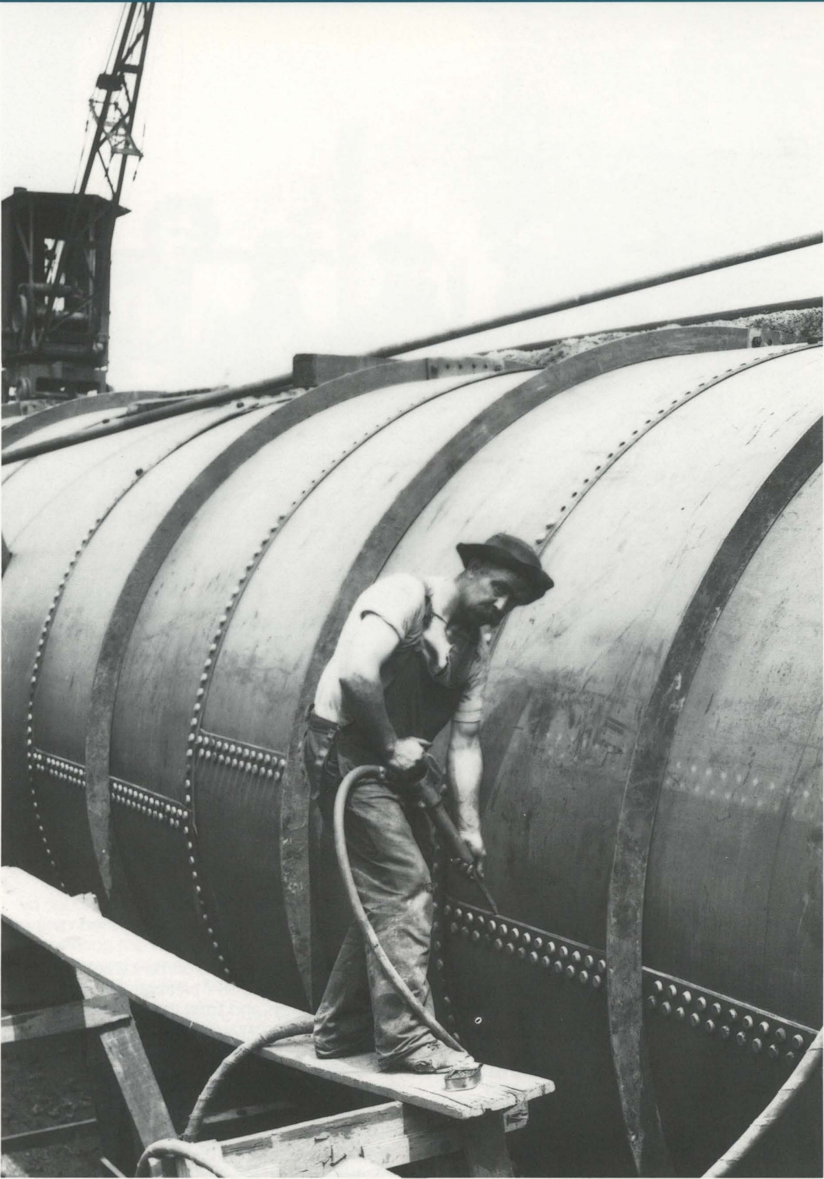
A workman is seen riveting one of the large steel conduits connecting the Torresdale filtration beds to the Lardner's Point Pumping Station.
