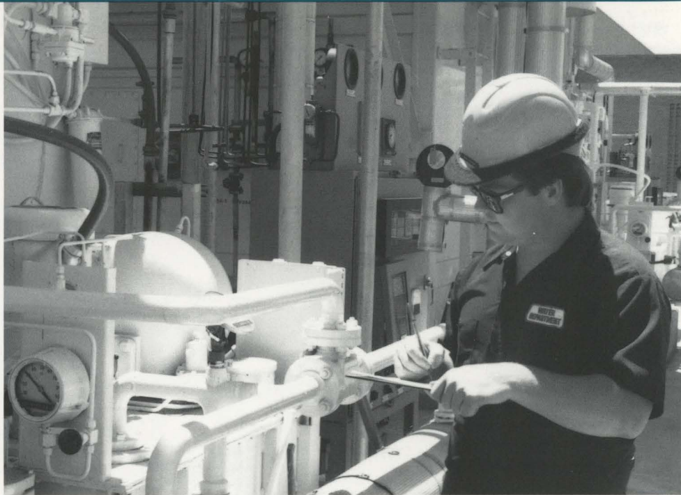
Operator checks 50 ton per day cryogenic fractional distillation units that supply oxygen to the covered aeration tanks at the Southeast Water Pollution Control Plant.
