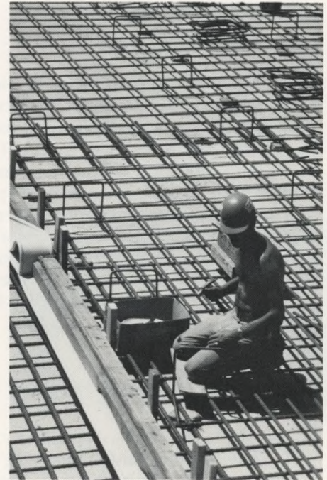
A workman completes installation of reinforcing steel for an aeration tank at the Southeast Water Pollution Control Plant.
