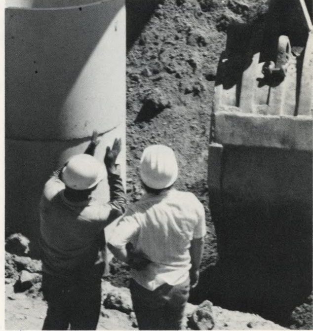
Engineers check the construction work for $10 million of improvements to the Queen Lane Water Treatment Plant.
