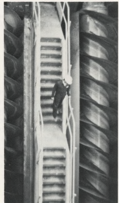
The Southwest Influent Pumping Station uses three of these 8.5 foot diameter, double helix, two stage screw pumps.
