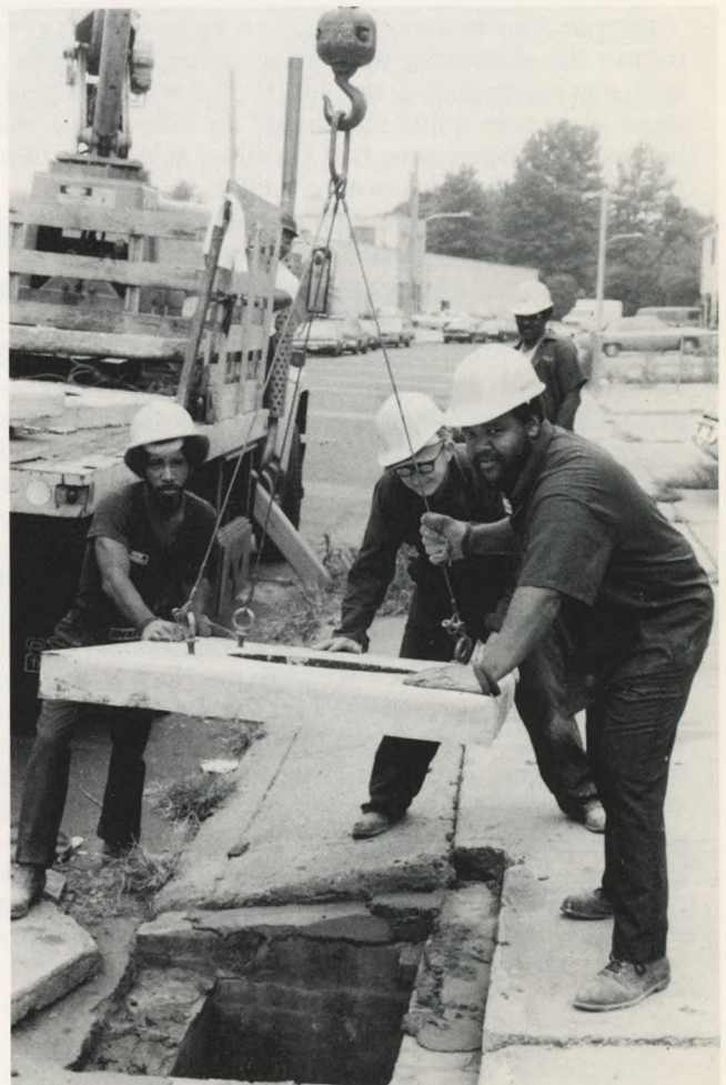
Sewer Maintenance crew replaces damaged slab at one of the 75,000 inlets in the City.
