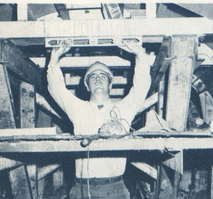
MAIN RELIEF SEWER: This huge tunnel sewer has spread two additional miles to relieve flooding in North Philadelphia. An engineer (above) checks out a portion recently completed.
