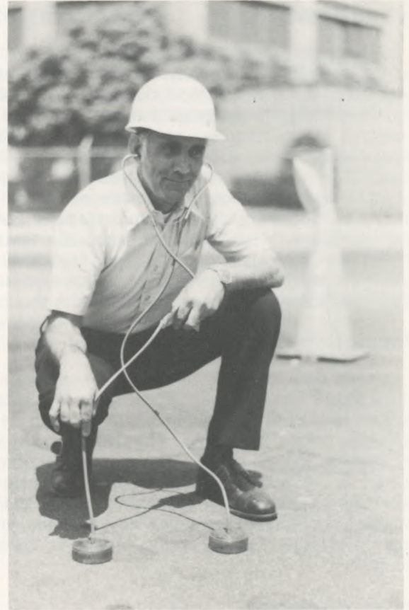
No, he is not listening to Mother Earth's heartbeat; Michael Elia, Water Distribution Supervisor, is using a geophone to detect the location of a water main leak.
