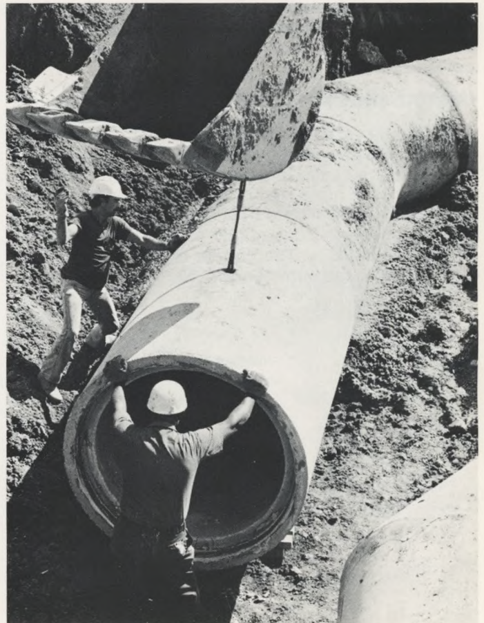
Contractors built 8 miles of sewers during Fiscal 1981 bringing the total sewer mileage to 2,927 miles.
