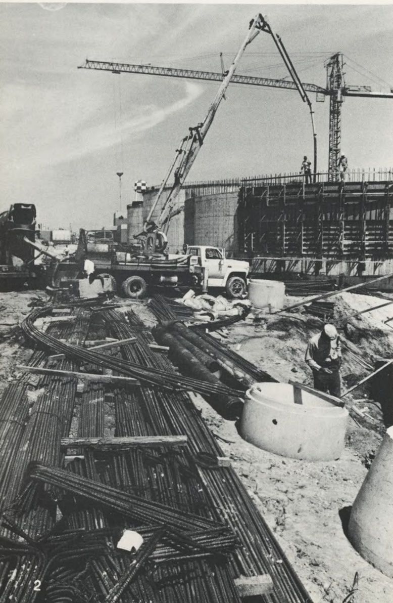
Each of the 8 new sludge digestion tanks built at the Southwest Plant is circular with a fixed cover and has an internal volume of over 2 million gallons.
