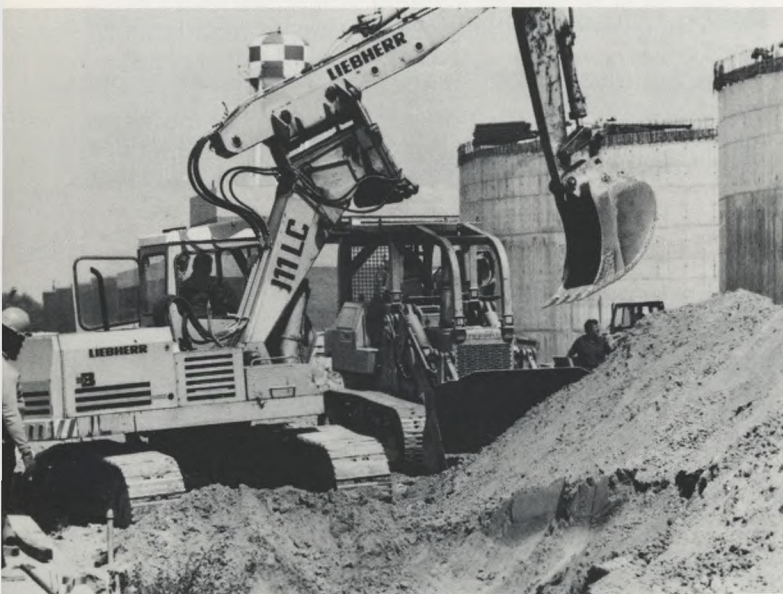
Over 75 contractors were involved in the construction of the $316 million Southwest Plant.
