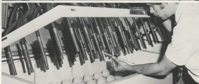
Stream Study: In an underground chamber in the Northeast, an engineer checks automated equipment that monitors storm water overflow into streams. During storms, the bottles fill automatically at pre-set intervals, and samples are later analyzed.
