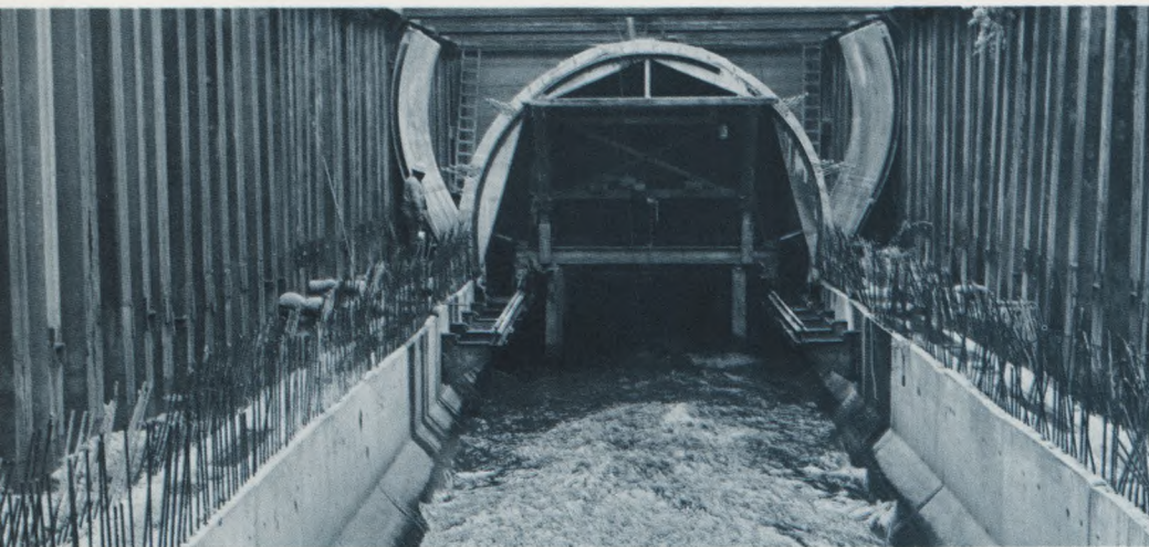
For Flood Control: The giant Mill Creek Sewer, which dates from the 1880's, was rebuilt for 272 feet in West Philadelphia.
