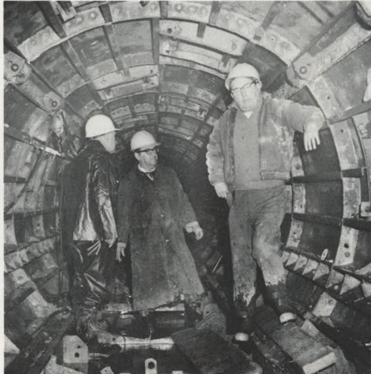
Tunnel Construction: Liner plates are ready for pouring of concrete. Plates can be moved from spot to spot.
