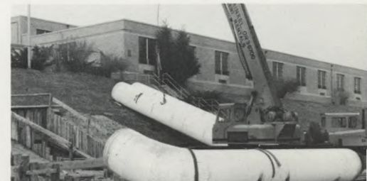
For Water Supply: Steel pipe, four feet in diameter, awaits placement at the Queen Lane Plant. It will carry water to consumers from a new reservoir.
