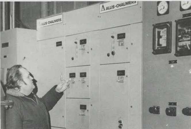
Automatic Controls: Operator checks some of the controls at the new Southwest grease incinerators.
