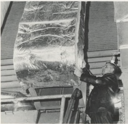
Maintenance: Thousands of vital jobs were performed by Building Maintenance men, ranging from ventilation to piping work.
