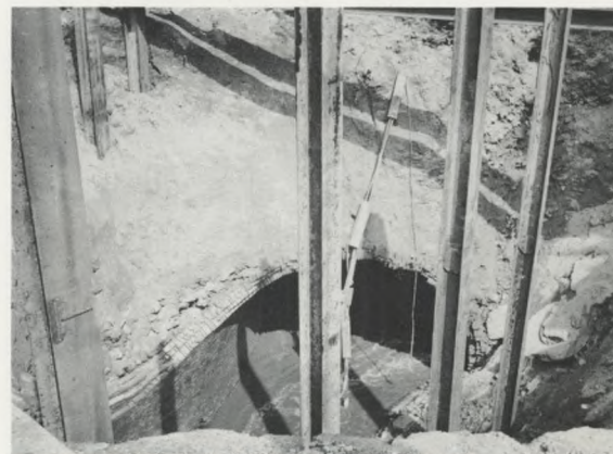
Sewer Collapse: In West Philadelphia, the giant Mill Creek Sewer collapsed for 70 feet. Built in the 1880's, it old bricks have been subject to increasing strains.
