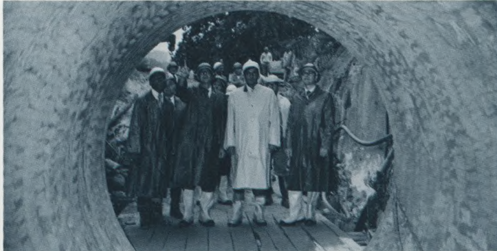
Engineering Marvel: Cut by boring machine through solid rock at depths of 50 to 100 feet, the new tunnel runs for 6,000 feet from the Schuylkill River. No blasting was necessary to cut the huge tube.
