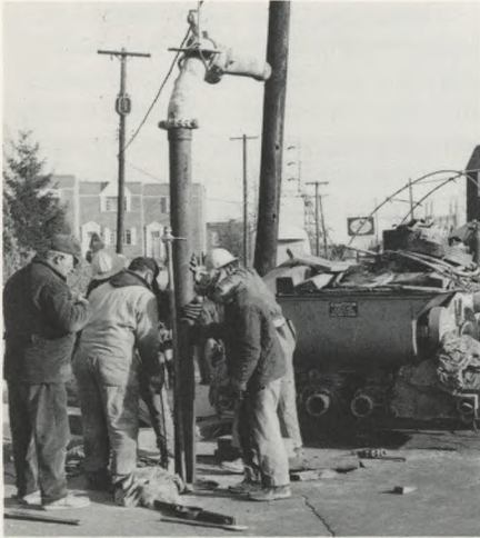
Pouring Concrete: Workmen lower a pipe, which will carry concrete to the tunnel 80 feet below. The concrete will spread behind tunnel liner plates to form a tube.
