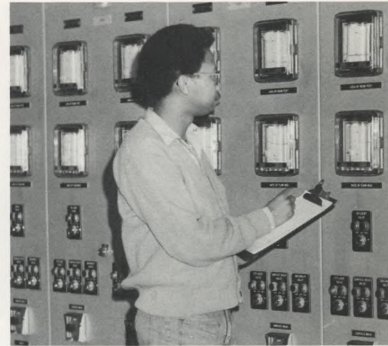
Central Control: Automatic and semi-automatic equipment regulates the treatment of water in all the city's plants. This panel controls filter beds at the Belmont Plant.
