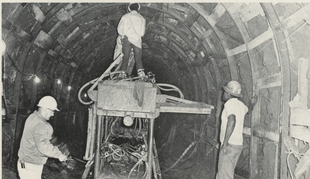
For Storm Flood Relief: The big Wakeling Street Relief Sewer was extended for another mile through Northeast Philadelphia. By September, 1971, it was diverting up to 2,000 cubic feet of storm water per second from overloaded sewers. Steel ribs are checked above, while top photograph shows finished concrete tube.
