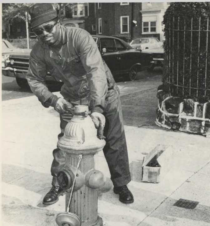
Locking Nut: Faced with the illegal opening of hundreds of fire hydrants on hot summer days, the distribution crews began to test a new type of locking nut on the top of some hydrants. The locking nut showed great promise in reducing water wastage.
