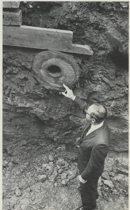
Historic Find: An old wooden water main, dating from the early years of the 19th century, turns up during digging on the east side of City Hall. Such mains, consisting of logs with bored centers, were abandoned by Philadelphia before 1850.
