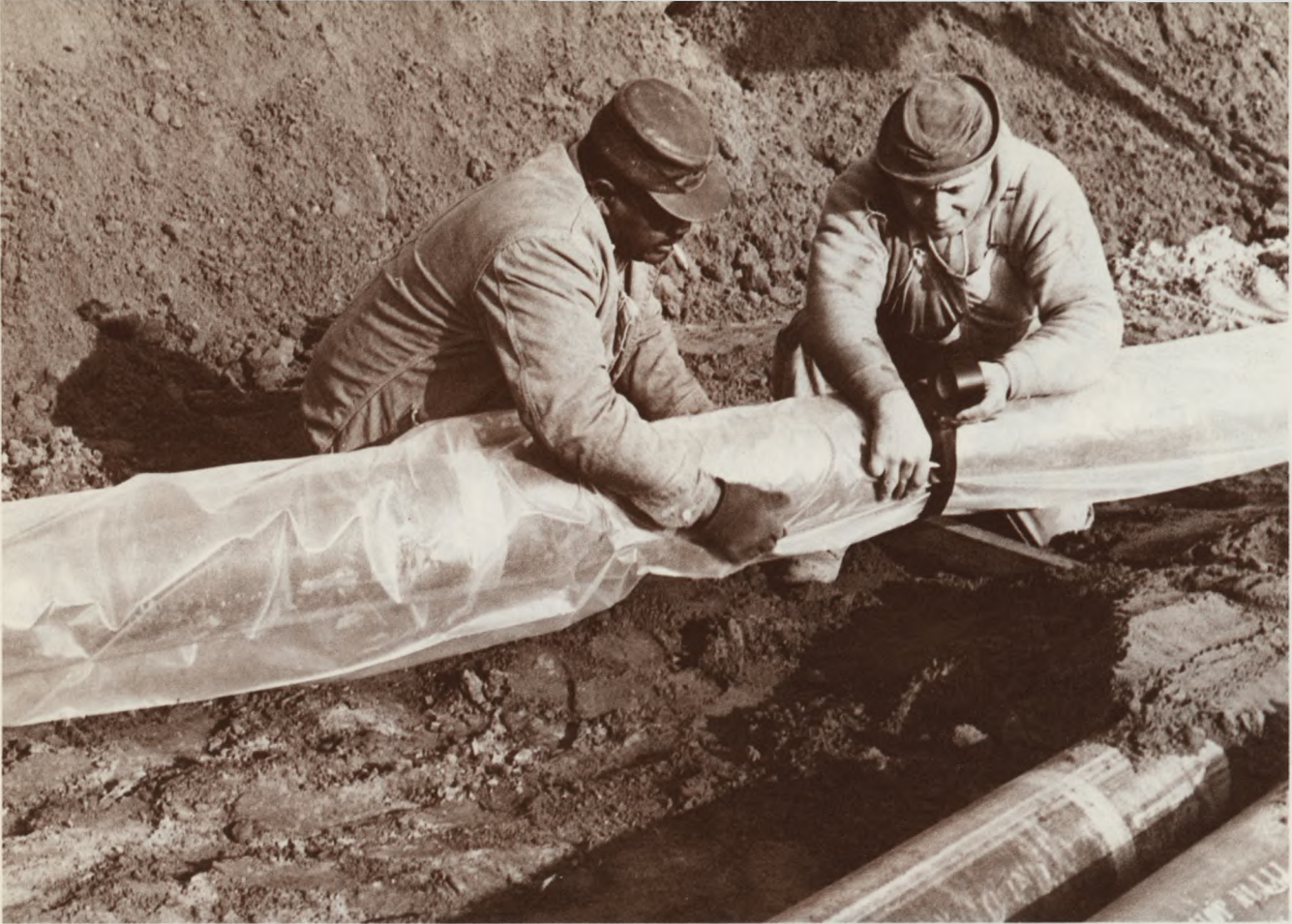
Polyethylene Protection: To protect new water mains against electrolysis, or deterioration from stray electrical currents, the Water Department began to wrap some of its mains in polyethylene before placing them in the ground. The main above was among several miles of new mains laid in Eastwick.
