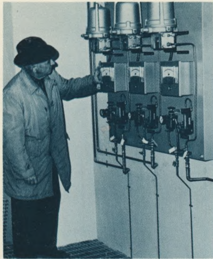
Measuring Feed: At the new Queen Lane chemical building, pneumatic devices will measure the rate at which carbon, alum and lime are applied to water.
