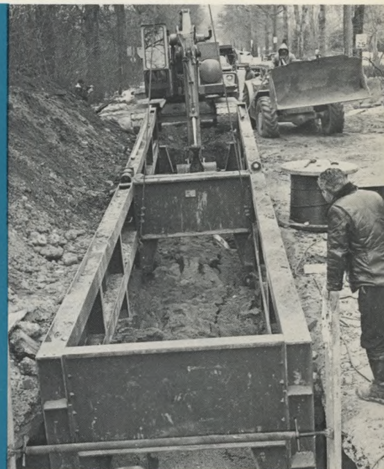
A new main was laid to carry Philadelphia water to Bucks County.
