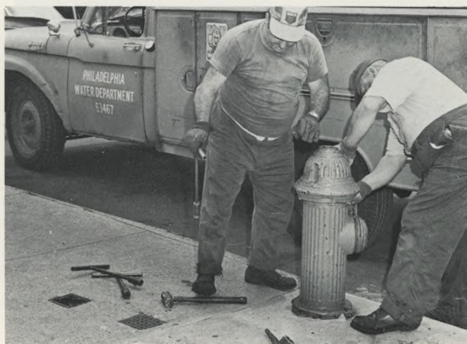
Fire Hydrant Repair: A good crew can disassemble the insides of a fire hydrant in a few minutes. Thousands of hydrant repairs are made each year, and thousands more hydrants are repainted. Hydrants are often inspected twice a year.
