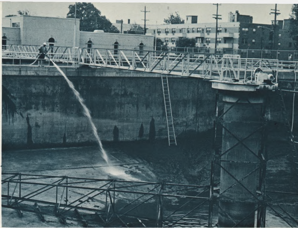
Spring Cleaning: Most of the basins, where water settles out its impurities, are cleaned twice a year at the treatment plants. At the Belmont Plant, 6,000 cubic feet of sediment was removed from settling and mixing basins in 1969 (above and right).
