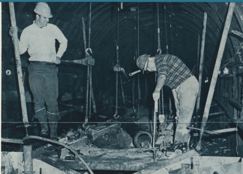
Another tunnel, 4,000 feet long, was added to a big storm relief sewer.
