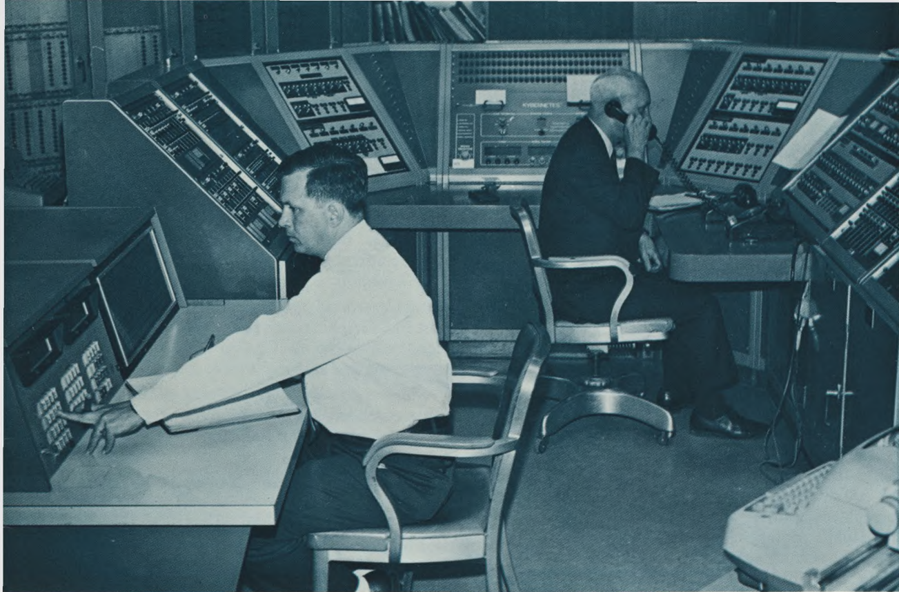
A computer (studied by operator at left) was installed at the Microwave Center to monitor water pumping stations and other facilities.
