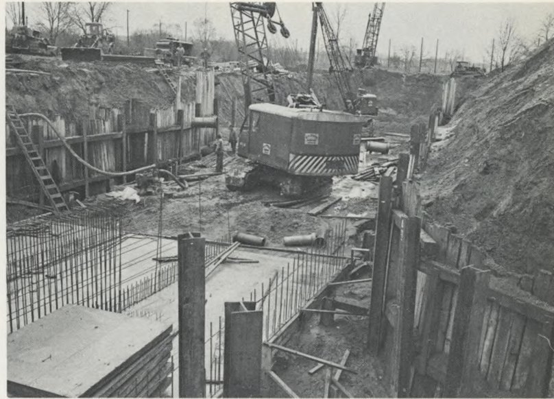
Sewers for Eastwick: Over 11 miles of sewers were built in Eastwick, an area which is being redeveloped in Southwest Philadelphia. The sewers included triple conduits (above and below) of reinforced concrete to pick up storm water or wastes.
