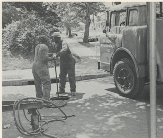
Valve Shut-off: Turning a large "key," workmen shut off a valve which controls flow through a water main. In 1968-69, distribution crews replaced 2,400 old valves and inspected 84,000 others.
