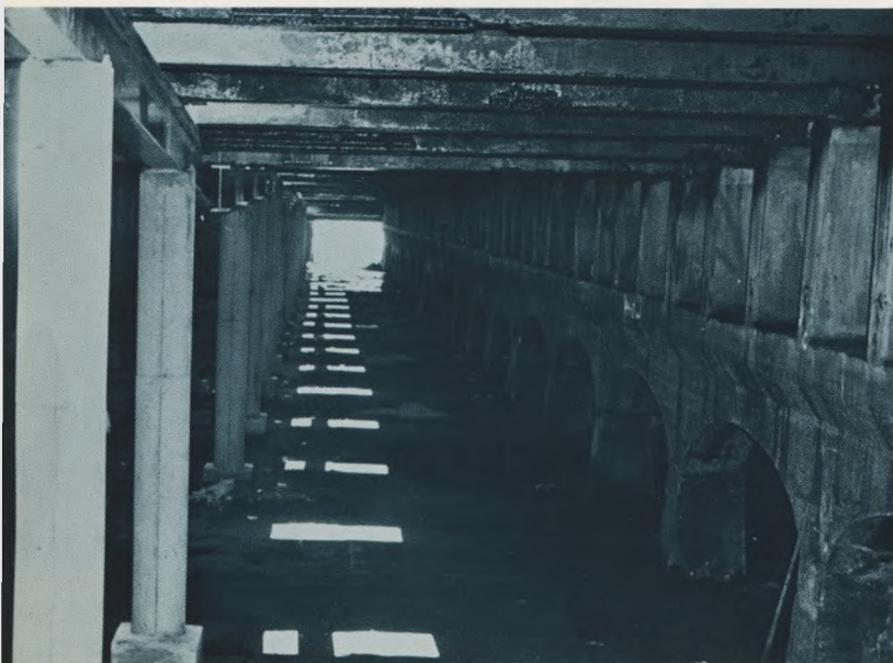
Future Reservoir: To provide space for storing 50 million gallons of purified water, workmen began to clear sand and gravel from 22 old filter beds at the Queen Lane Plant and to make modifications in them. One of the cleared beds above.
