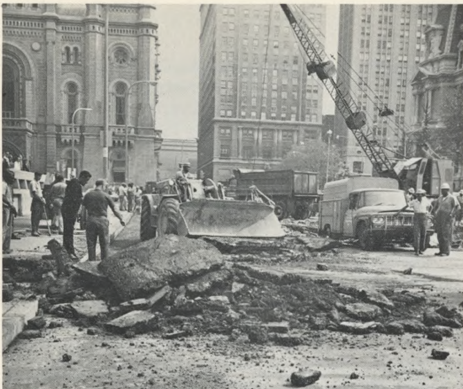
Water Main Break: Every day is an emergency for distribution crews, for water main breaks average two or three a day. In 1968-69, there were more than 1,900. This break occurred across from City Hall.
