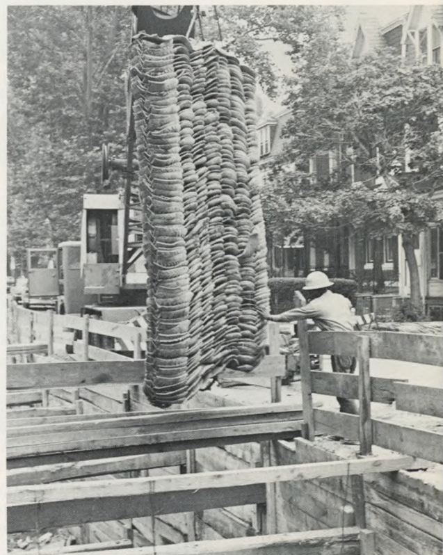
A New Use for Old Tires: At the point where the completed tunnel is being tied into tributary sewers, a tire blanket is lowered to deaden the effects of blasting. Truck at left holds concrete for the job.
