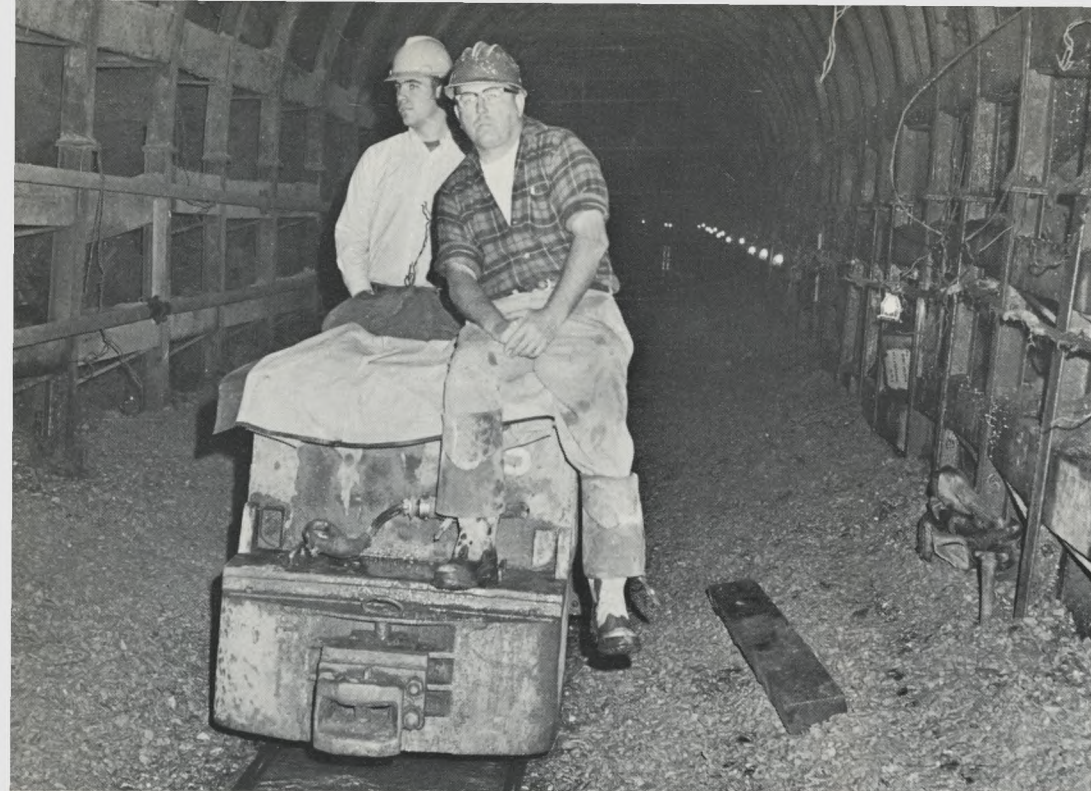
Final Stage: The most recent segment of the Main Relief Sewer went into service late in 1969. A 10-ft. concrete tube in tunnel, it extends along Sedgley Avenue and 16th Street and was built at a cost of $1.7 million.
