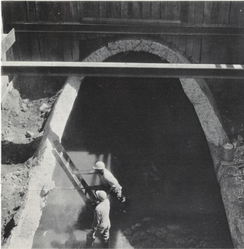
Old Sewer: Two-thirds of the storm flow from the old Wakeling Street Sewer (left) will be diverted into the new Relief Sewer, which runs two miles from the Roosevelt Boulevard to the Delaware River.
