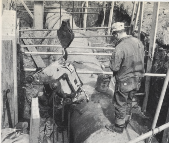
Water Main Repair: The repair of broken water mains was an almost daily occurrence in 1962 as 963 mains snapped. Using a powered cutting tool, maintenance men (photo) prepare to cut away a section of a large main which has cracked.
