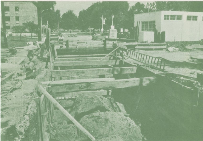
Last Lap: A chamber constructed near Roosevelt Boulevard to divert storm flow from the old Wakeling Street Sewer formed the last link in the new Relief Sewer, which was almost complete by the end of the year. The new sewer will relieve storm flooding in Frankford and nearby areas.
