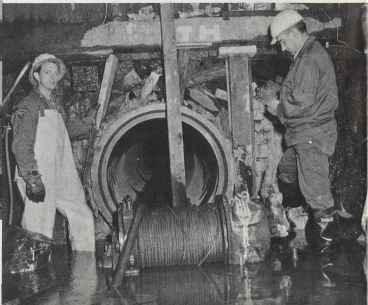
For Cleaner Rivers: Big interceptor sewers to divert sewage away from the rivers to sewage treatment plants were further extended. A branch sewer (below) enters a huge interceptor under construction on the west bank of the Schuylkill River.
