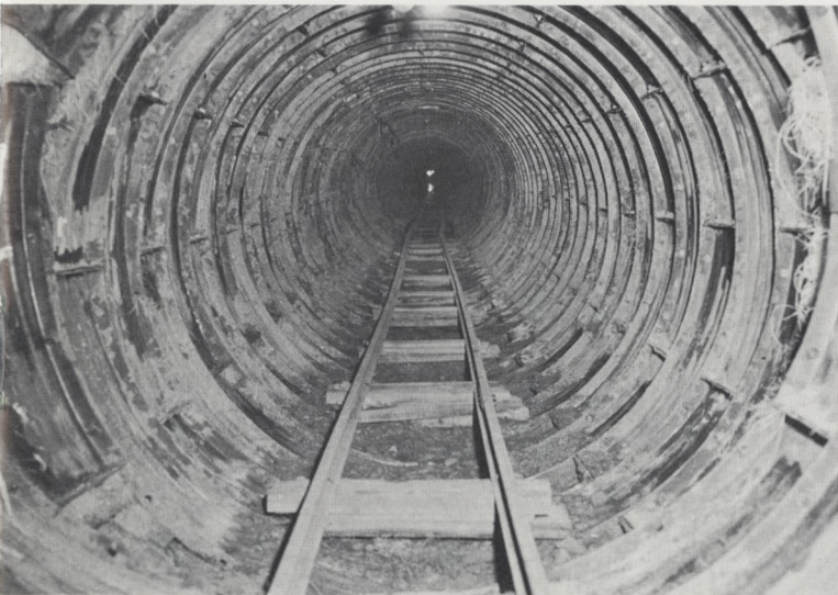
Schuylkill Clean-Up: Final clean-up of the lower Schuylkill River was in sight as another link was built in a long intercepting sewer on the west bank. The sewer will carry sewage to the Southwest Sewage Treatment Works.
