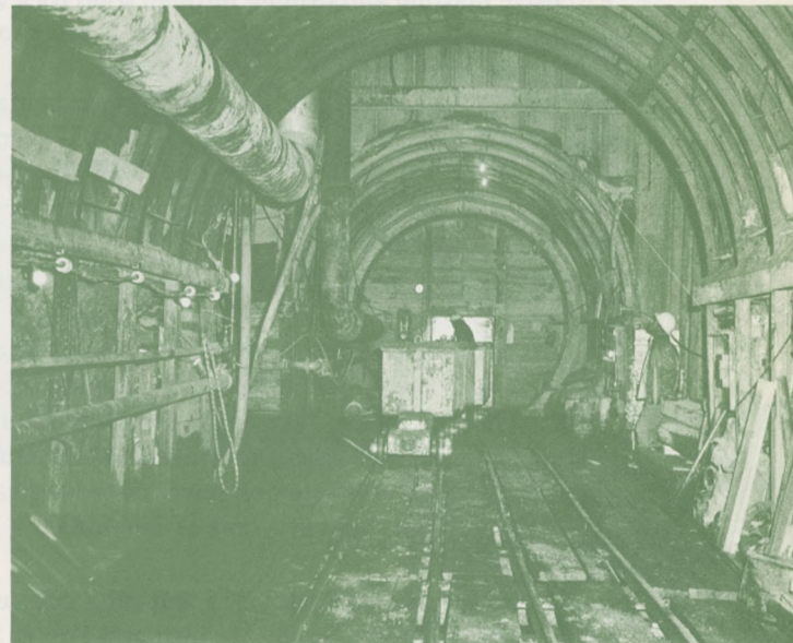
Air Lock: Cars enter a compressed air lock, built to protect workmen against water seepage and loose soil. Tunneling was an engineering feat because of difficult soil and rock.
