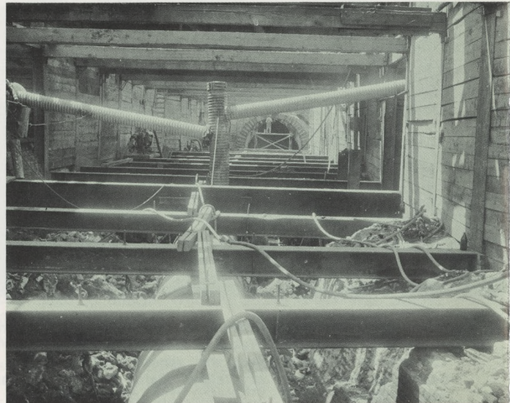
Mill Creek Sewer: To relieve storm flooding in West Philadelphia, part of the old Mill Creek Sewer was rebuilt in 46th Street north of Market at a cost of nearly $1 million.
