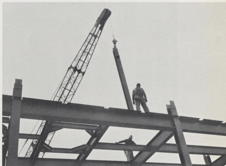
New Plant: A crane swings a steel beam into place for the rising pre-treatment building. Modern chemical-feeding devices in the new building will greatly improve the efficiency of water treatment.
