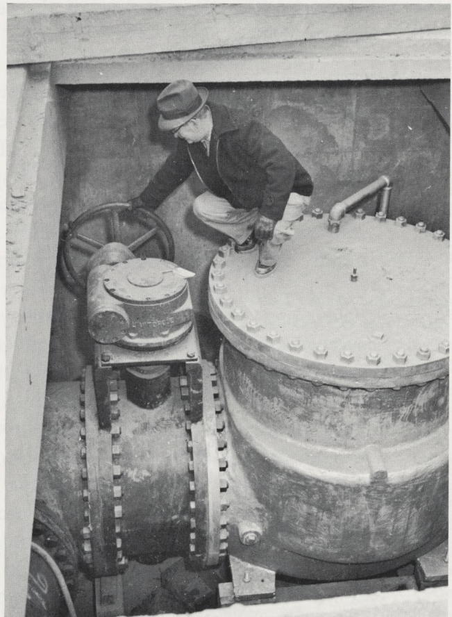
This giant altitude valve was but a small part of the intricate underground pipework and controls built during the year at the new Belmont Water Treatment Plant.
