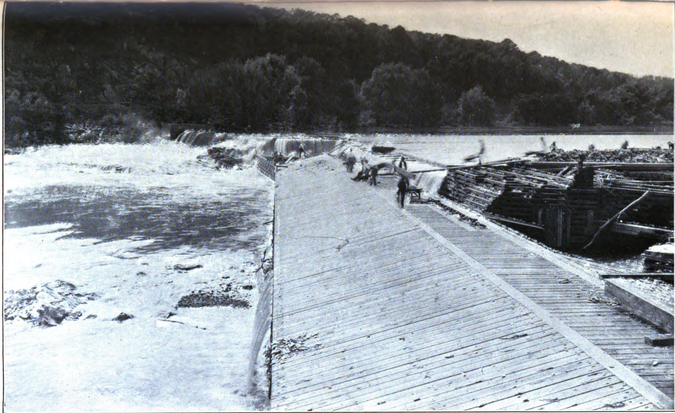
NEW DAM PARTLY FINISHED IN FRONT OF THE OLD STRUCTURE AND VIEW OF CRIBBING CONSTRUCTED ACROSS THE BREAK IN THE OLD DAM.
