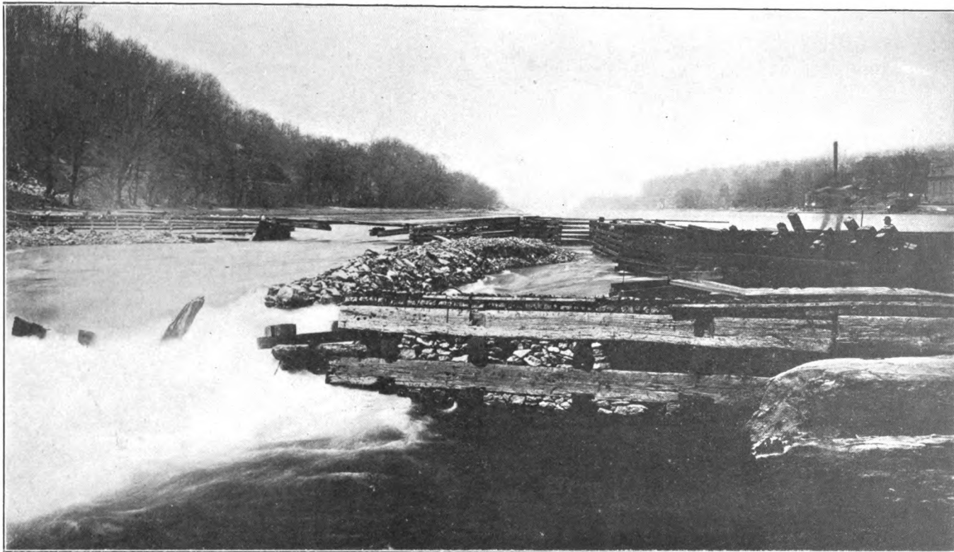
FLAT ROCK DAM, SHOWING PARTLY FINISHED TEMPORARY CRIBBING TO SHUT OFF THE WATER WHILE REPAIRING THE BREAK IN THE DAM.
