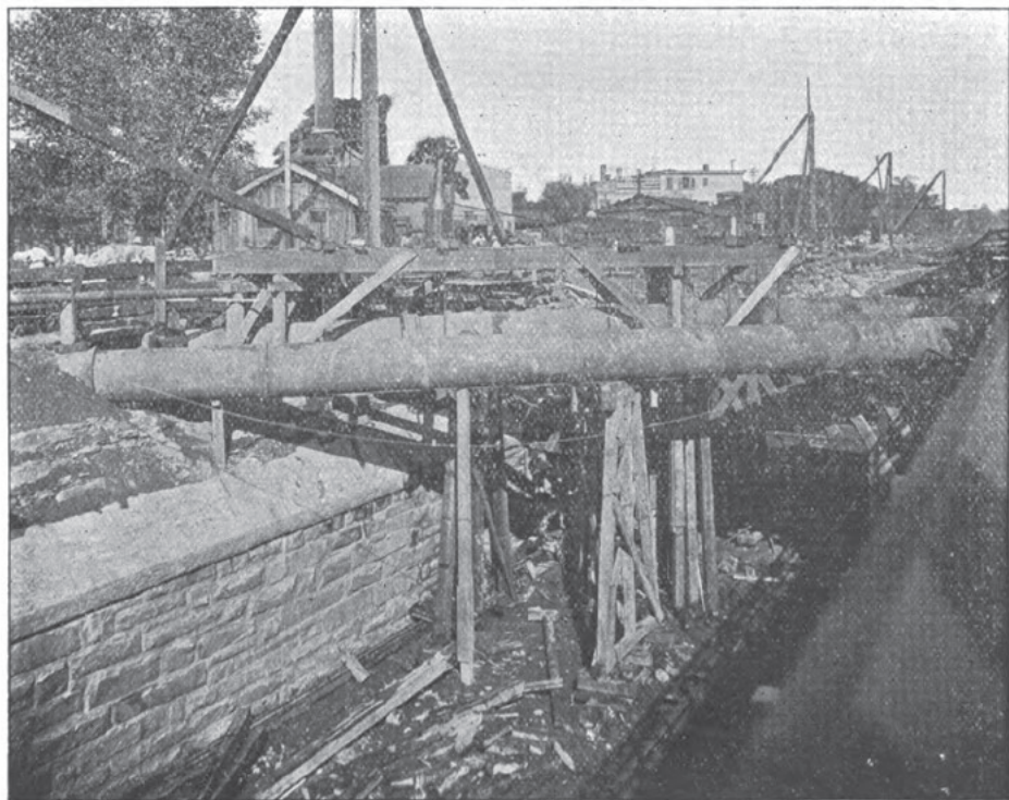
V IEW AT TWENTY-FOURTH STREET AND PENNSYLVANIA AVENUE SUBWAY, S HOWING METHOD OF SUPPORTING 48 INCH MAINS.
